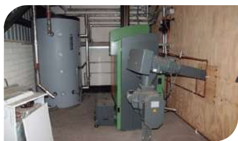
Figura 2 Caldeira de aquecimento a biomassa (Statfold Barn Railway - biomass heating system by Chris Allen, CC BY-SA 2.0 < https://creativecommons.org/licenses/by-sa/2.0 >, via Wikimedia Commons).
